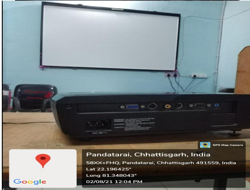
Figure — System Projector computer's installed in facility
