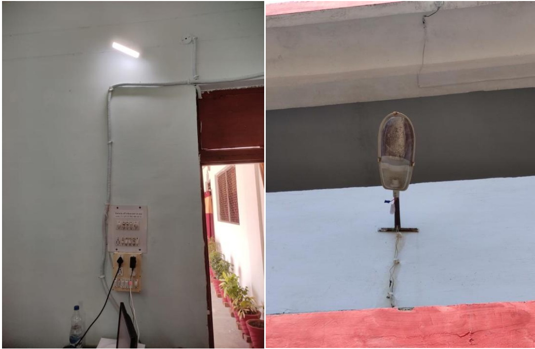
Figure - LED lights installed in facility
