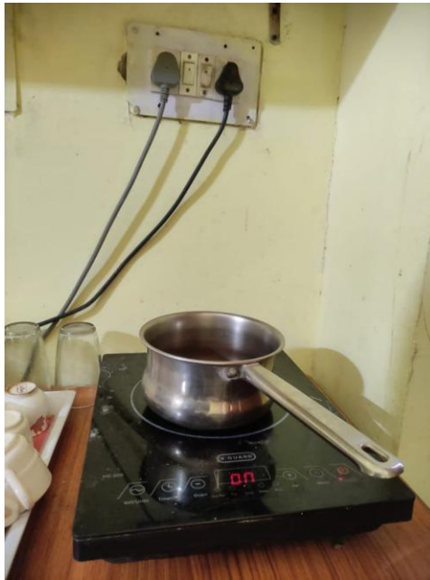
Figure - Induction Oven installed in facility
