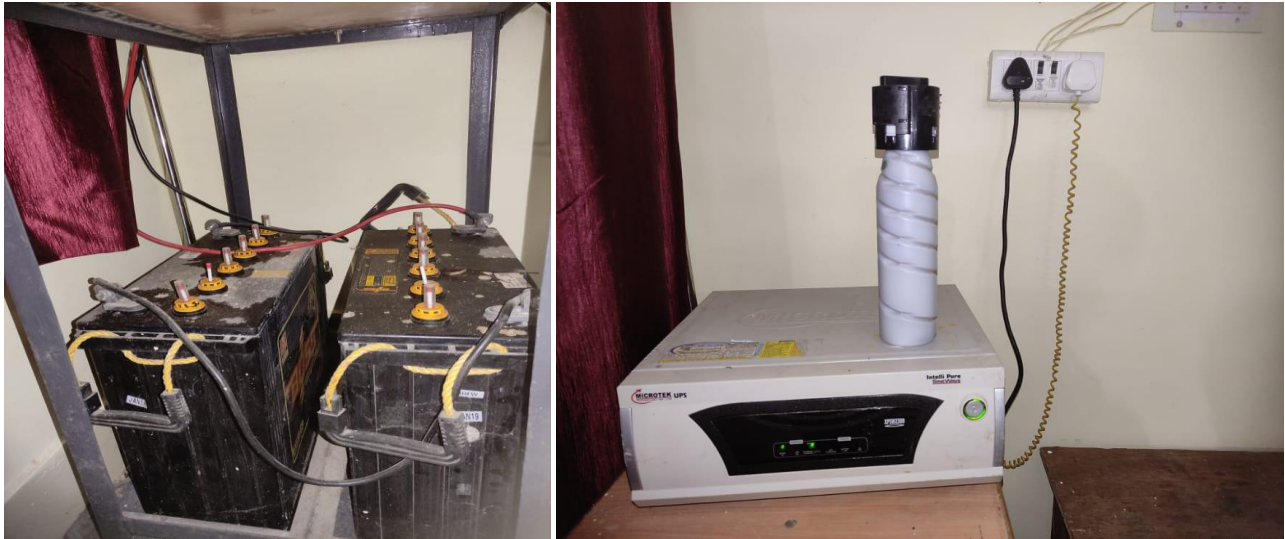
Figure - show battery installed in facility Uninterruptible Power Supply
