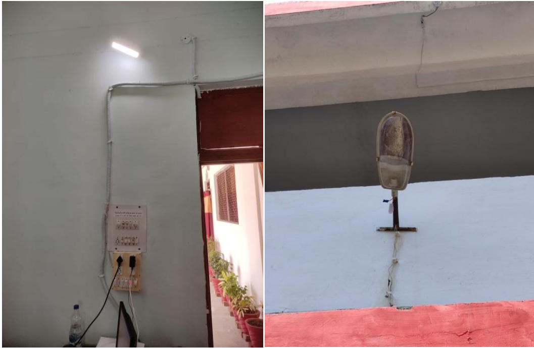
Figure - LED lights installed in facility
