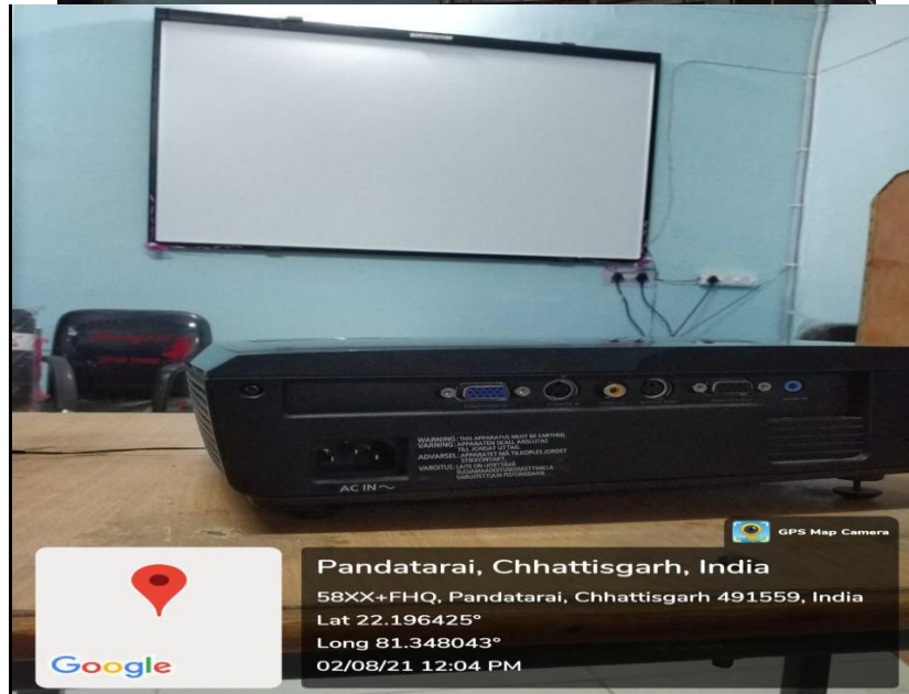
Figure — System Projector computer's installed in facility
