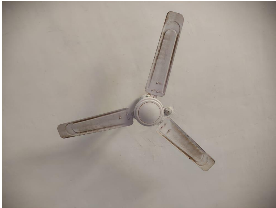
Figure - Ceiling Fans installed in facility
