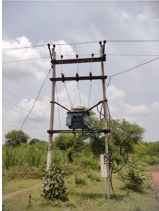
Figure - Transformer installed in facility
