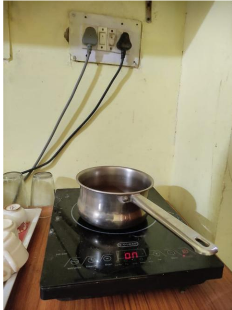
Figure - Induction Oven installed in facility
